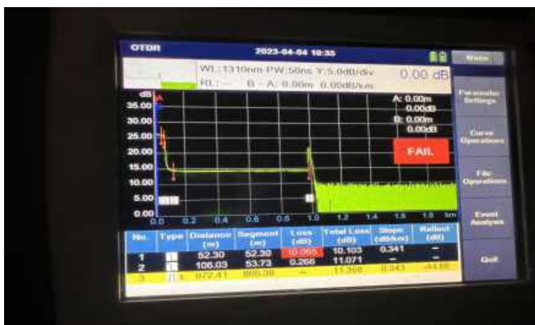
Link trace and fault finding
